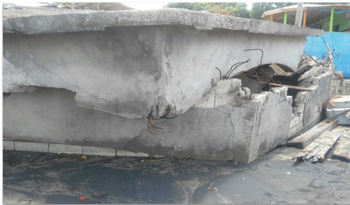
Figure 5. Collapsed fish-cleaning structure.
