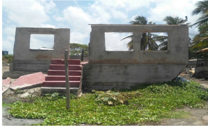
Figure 3. Structure damaged by Hurricane Ivan.
