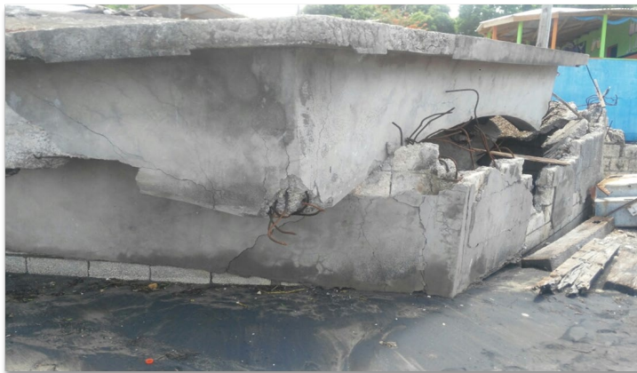
Figure 5. Collapsed fish-cleaning structure.
