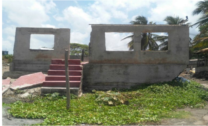
Figure 3. Structure damaged by Hurricane Ivan.
